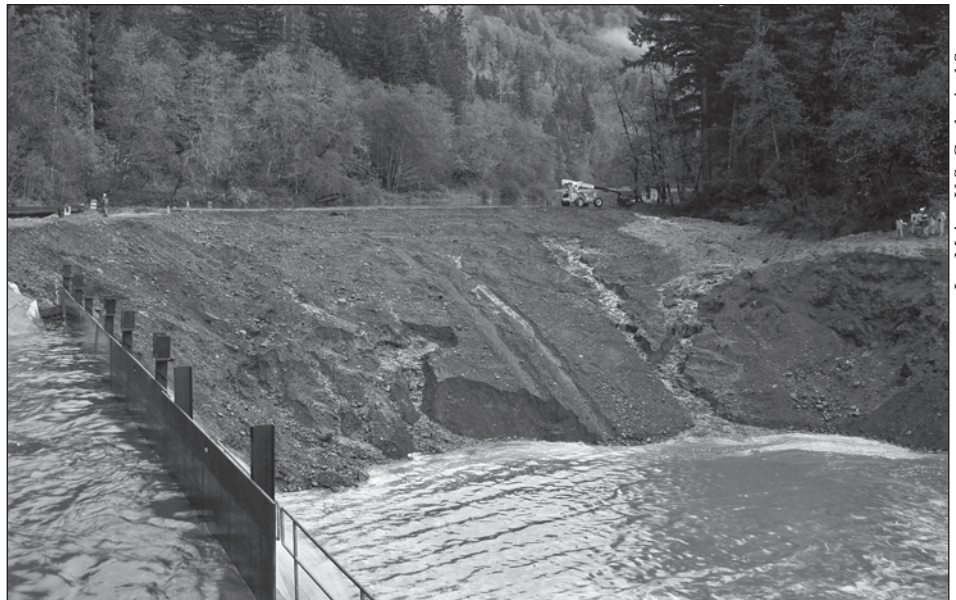
As the river rose on October 19, 2007, the earthen cofferdam became saturated and seepage erosion and mass failures appeared on the dam face.
