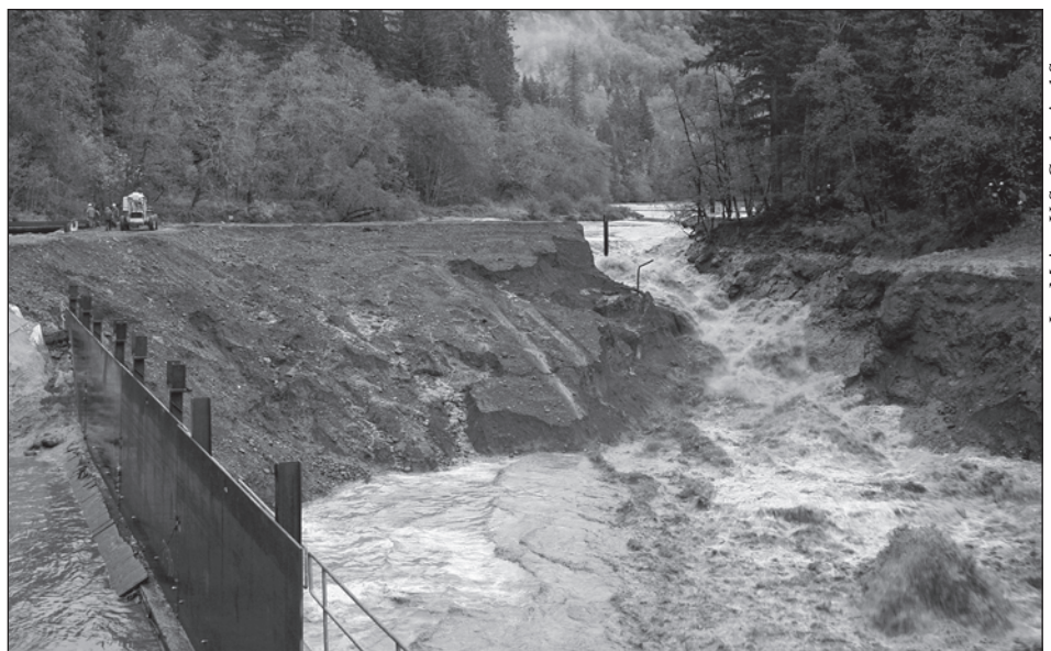
Less than an hour after the cofferdam was notched, the breach channel had rapidly expanded and was actively eroding the cofferdam.
