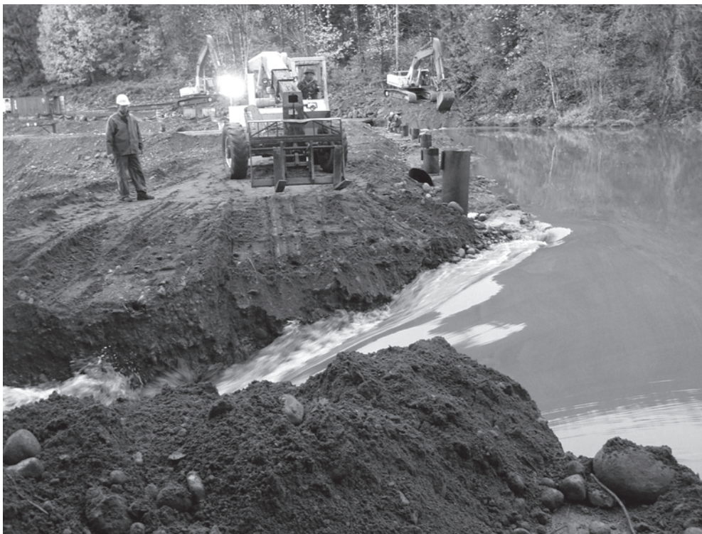
Dismantling Marmot Dam on the Sandy River, Oregon, improved river access for fish and provided valuable information about how a river system responds to dam removal. Above, crew breach the cofferdam that held back the river while Marmot Dam was removed.
