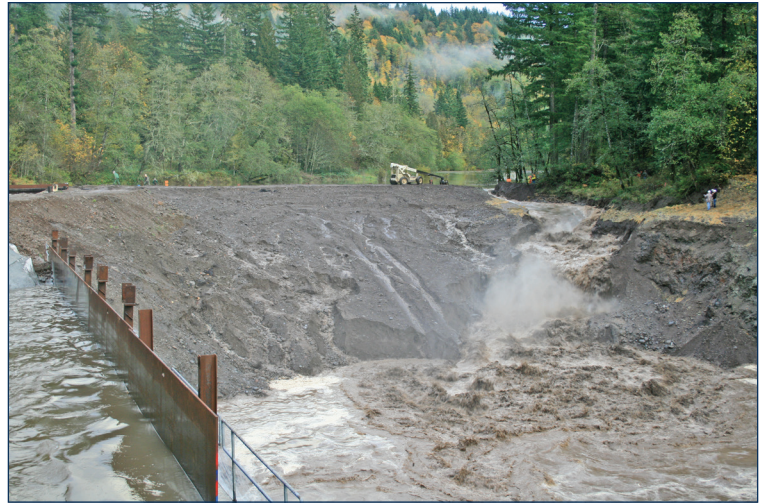
The 2007 breaching of the Marmot Dam on the Sandy River, Oregon, released about 20 million cubic feet of accumulated sediment. About 60 percent of it was deposited downstream within 2 years. Above, the knickpoint emerges in the earthen cofferdam that was built to allow workers to remove the concrete infrastructure.
