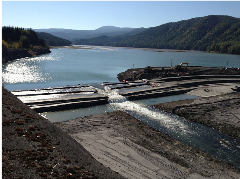
Figure 8. Pilot raise of the Sediment Retention Structure (SRS) spillway under construction during summer 2012. [Colour figure can be viewed at wileyonlinelibrary.com ]
