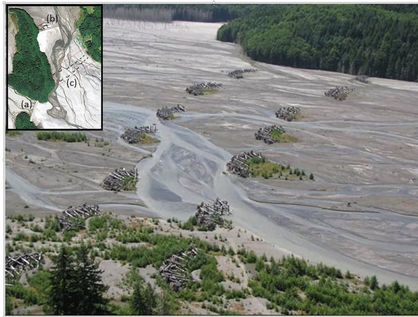
Figure 7. Grade building structures installed in the 2010 Pilot Project. Inset orthophoto shows (a) cutoff berm, (b) cross-valley step-weir and baffle structure, and (c) island building structures. Main picture shows Engineered Log Jam island building structures in area outlined in red in the orthophoto three years after their installation. [Colour figure can be viewed at wileyonlinelibrary.com ]
