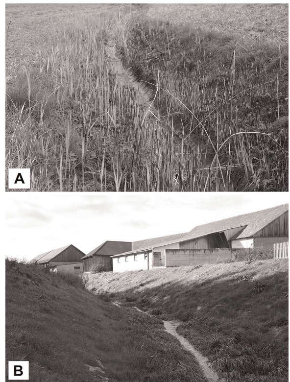
Fig. 6. Channel protection structures: (A) Concrete chutes along the Kaja River downstream of Dam 7 (refer to Fig. 2B); (B) Rip raps (partially covered by grass) along the Fugnitz River upstream of Dam 7 (refer to Fig. 2B).
