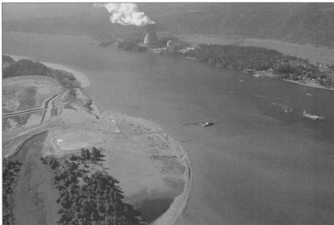
Pipeline and hopper dredges at work removing sediment clogging the shipping channel in the Columbia River below the Trojan nuclear power plant on the Oregon shore.
