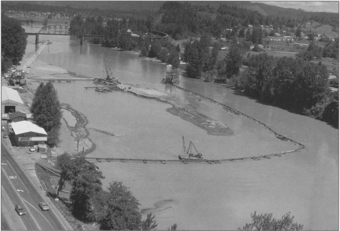
A pipeline dredge at work on the Toutle River, vacuuming material from the river bottom and moving it through the pipeline to shore for disposal.
