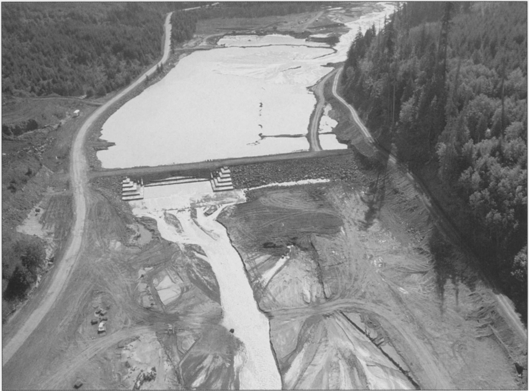
The Corps built this retention structure on the South Fork Toutle River to trap debris, which was then excavated and removed to disposal areas away from the river.
