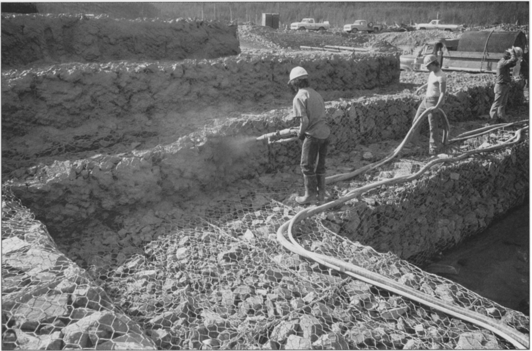
Workers spraying the cement slurry on the rock-filled gabions forming the spillway of one of the temporary debris dams constructed on the forks of the Toutle River.
