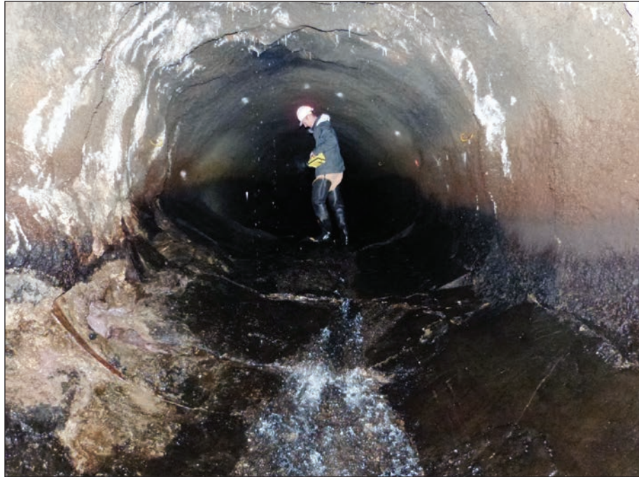
Figure 4-2—Location where tunnel floor had heaved. Note offset in tunnel floor from where person is standing to water flow in foreground (from Britton et al. 2016).
