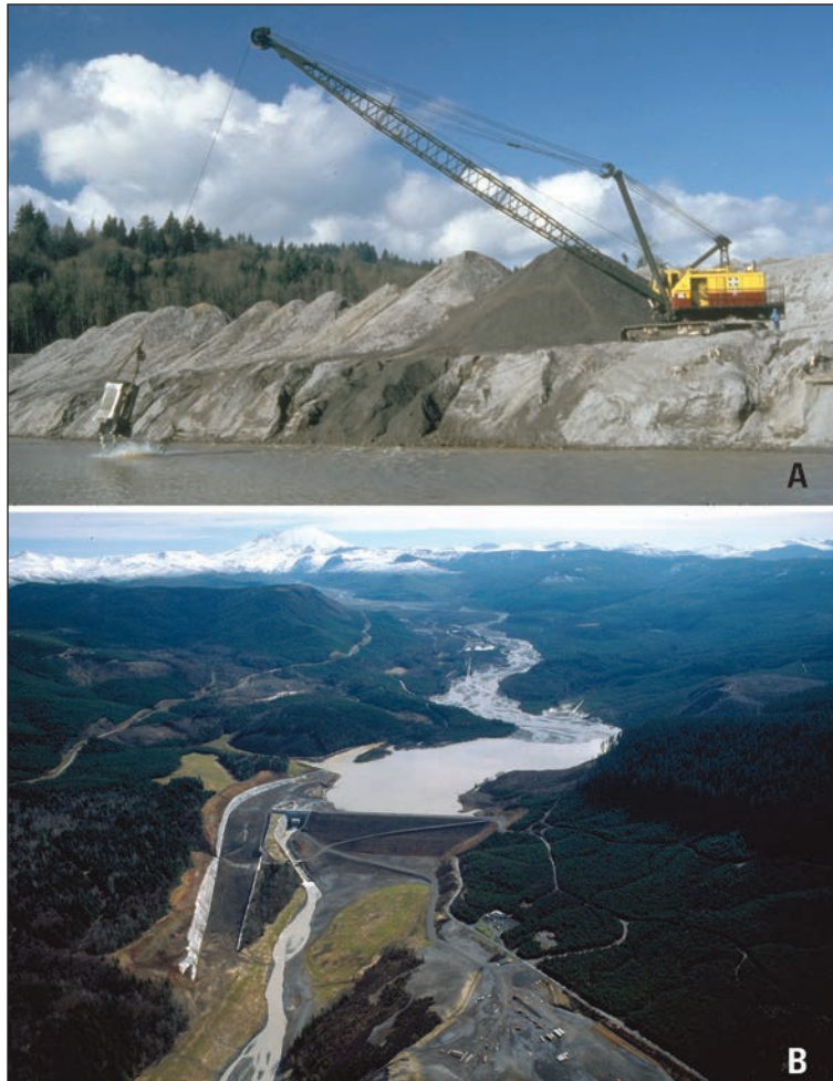
Figure 2-18—Mitigation of post-1980 sediment transport along the Toutle-Cowlitz River system. (A) Sediment dredging along Cowlitz River. U.S. Geological Survey, February 2, 1981. (B) Oblique aerial view to east of sediment retention structure constructed on North Fork Toutle River valley. Photo by Bill Johnson, U.S. Army Corps of Engineers. Source: Major et al. (2005).
