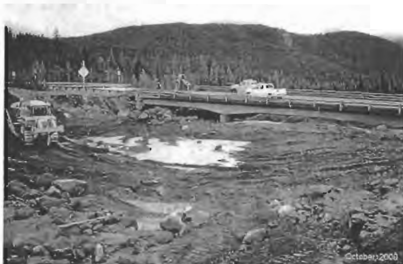
Figure 16. Oregon Department of Transportation highway crews clearing sediment beneath the OR 35 bridge over the White River. Lahars, generated by intense rain in October 2000, filled the river channel and damaged the bridge.
